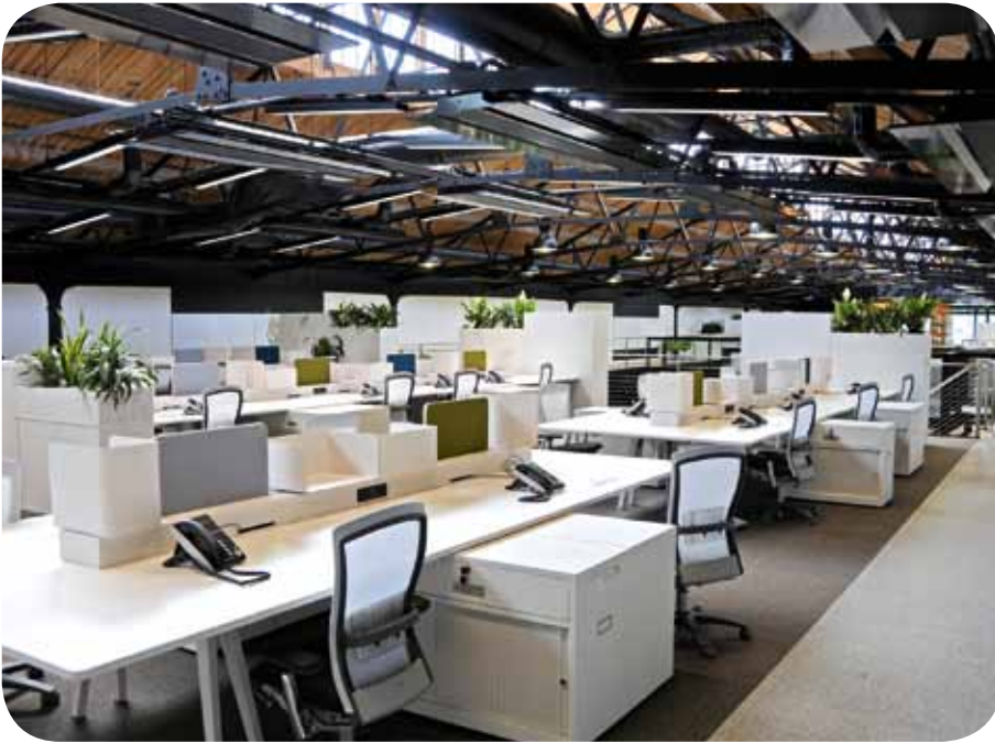
The Chilled beams are a valuable piece of engineering kit, but also make building occupants think about the space they inhabit. Pic: Angelo Marcina
